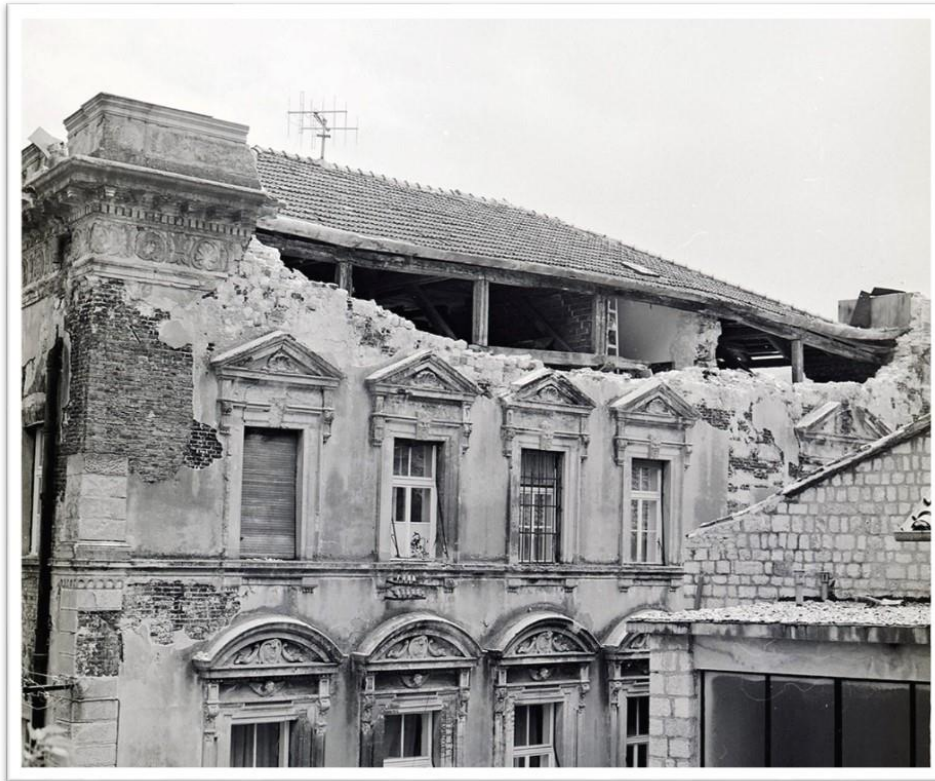
Crnogorski zemljotres 1979. - stari grad Kotor. Montenegro 1979 earthquake - Kotor Old town.
