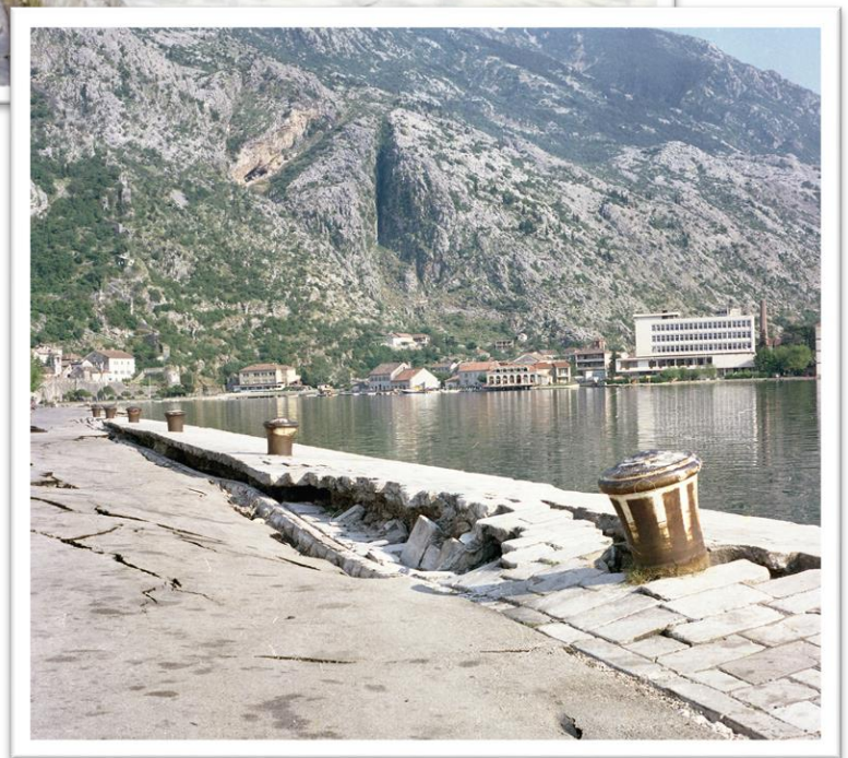
Crnogorski zemljotres 1979. - srušeni hotel Fjord i pogled na oštećenu kotorsku rivu Montenegro 1979 earthquake – Kotor, Hotel Fjord and damaged seafront.
